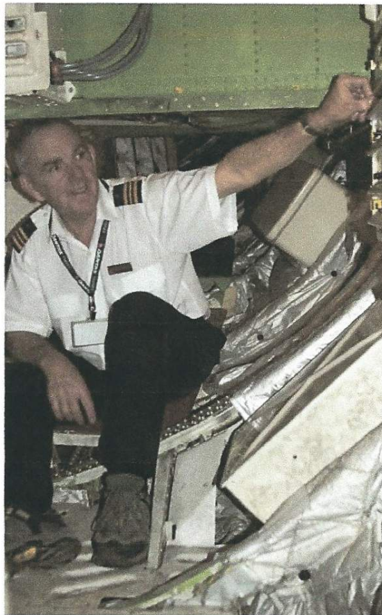
● Engineer Roger Blakey inside the main equipment centre. OWEN ZUPP
